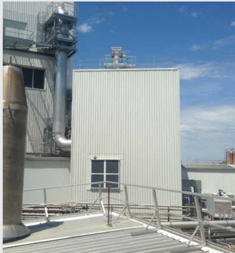
MSD1 Dryer Stack post baghouse installation – no visible emissions.
