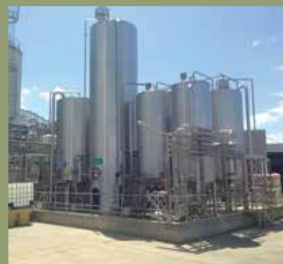
New Separators and Lactoferrin CIP Kitchen infrastructure located in Central CIP Facility.
